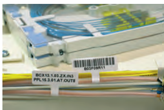
Fibre optic cable markers
