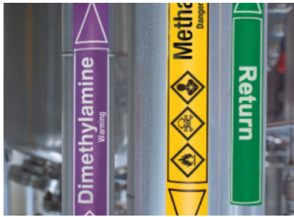
Pipe & valve marking
